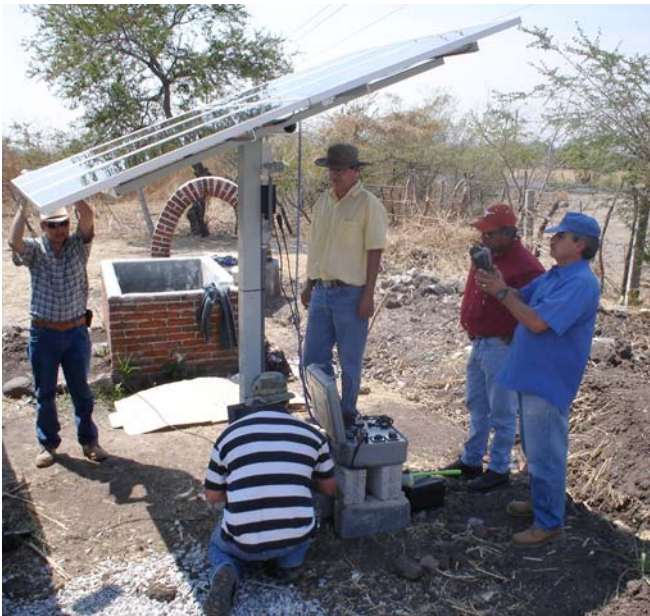
Fig. 2. Huitchila PV Array in Las Margaritas under test by UNAM, NMSU, and FIRCO personnel.
