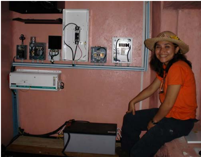
Fig. 5. COHCIT Sosoal PV satellite telecenter with internet connectivity using quality BOS components with SOLARIS installer Ethel Enamorado in Lempira, Honduras (2004).
