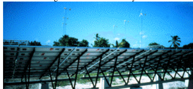
Fig. 9. Xcalak, Mexico wind turbines and PV array (1993).
