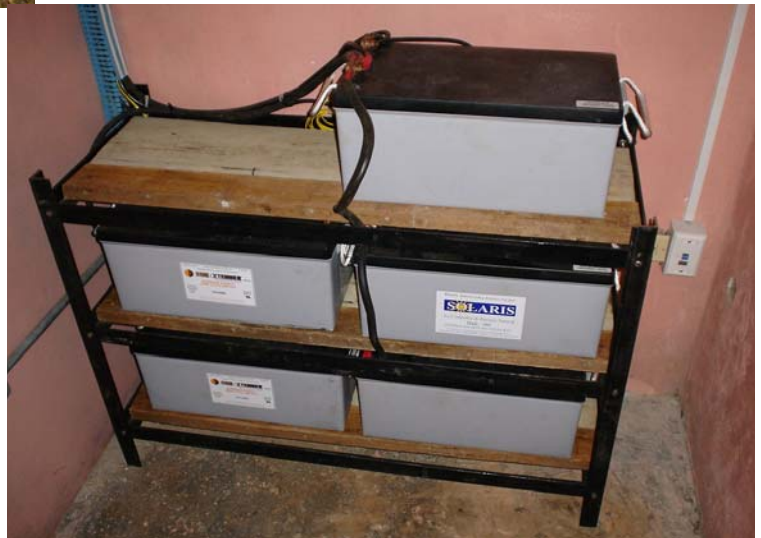
Fig. 9. Concorde SunExtender AGM batteries with 1290 Ah capacity for Sosoal telecenter.
