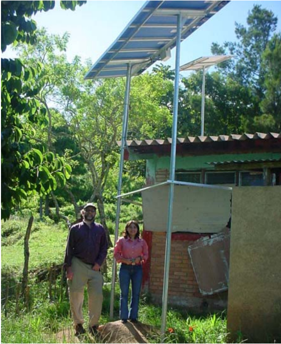
Fig. 2. Montaña Grande 600 Wp PV array. The PV array is connected through a listed Trace TCB6 PV Source Circuit Combiner box, with each string leg fused. Two Square D 30 A AC breakers rated at 120/240 V are used as a disconnect for the PV array; this represents about 17 A per leg of dc power from the modules.
