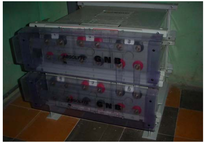
Fig. 3. GNB sealed batteries providing 800 Ah of energy storage at 12V for the Montaña Grande school complex.
