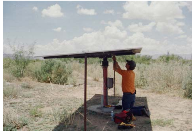
Fig. 1: FIRCO engineer conducting performance evaluation of an 8-year old PV water pumping system at Rancho Jeromín, Chihuahua.
