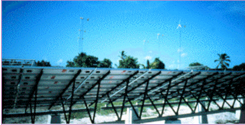
Figure 2. Xcalak wind turbines and PV array in Quintana Roo, Mexico.
